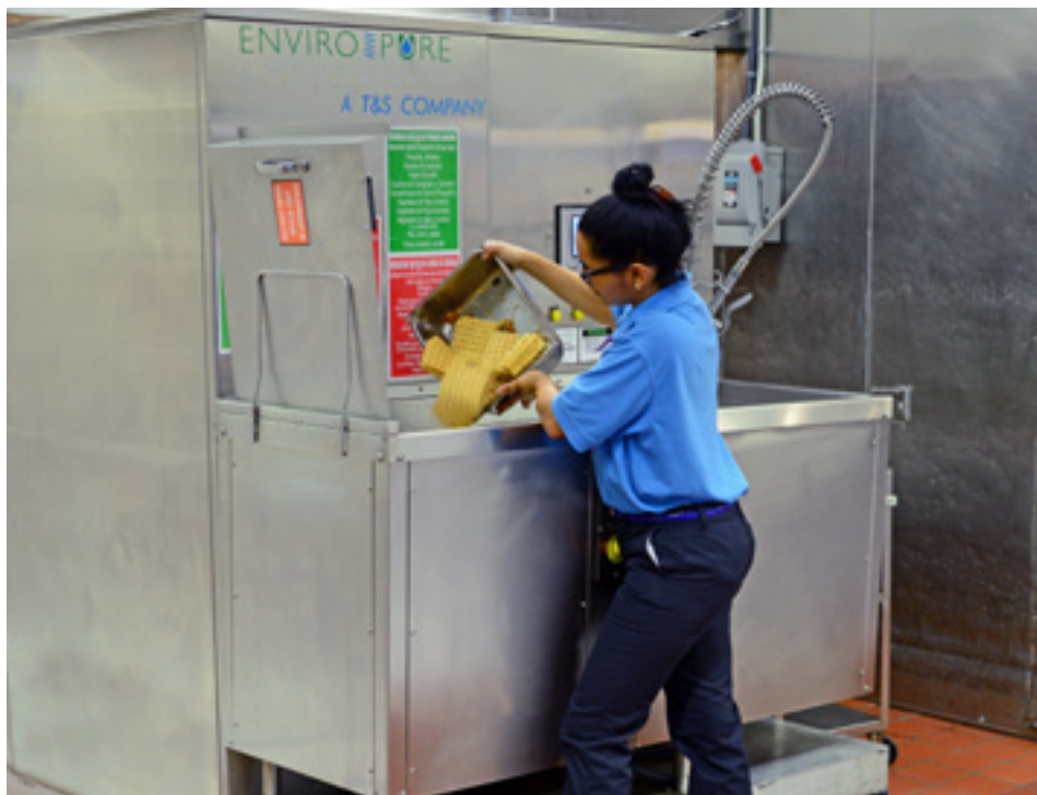
Biodigesters conveniently located in New Rochelle Hospital's kitchens allow the facility to repurpose food waste into gray water.
