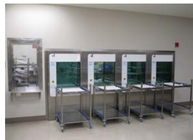
Four Belimed WD 290s wash/disinfectors clean over 450,000 instruments per month.
